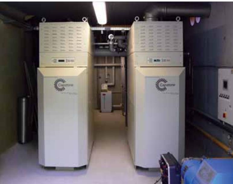
The cogeneration system generates 1 million kWh of electricity and 1.8 million kWh of thermal power onsite, exceeding 80 percent energy efficiency.
